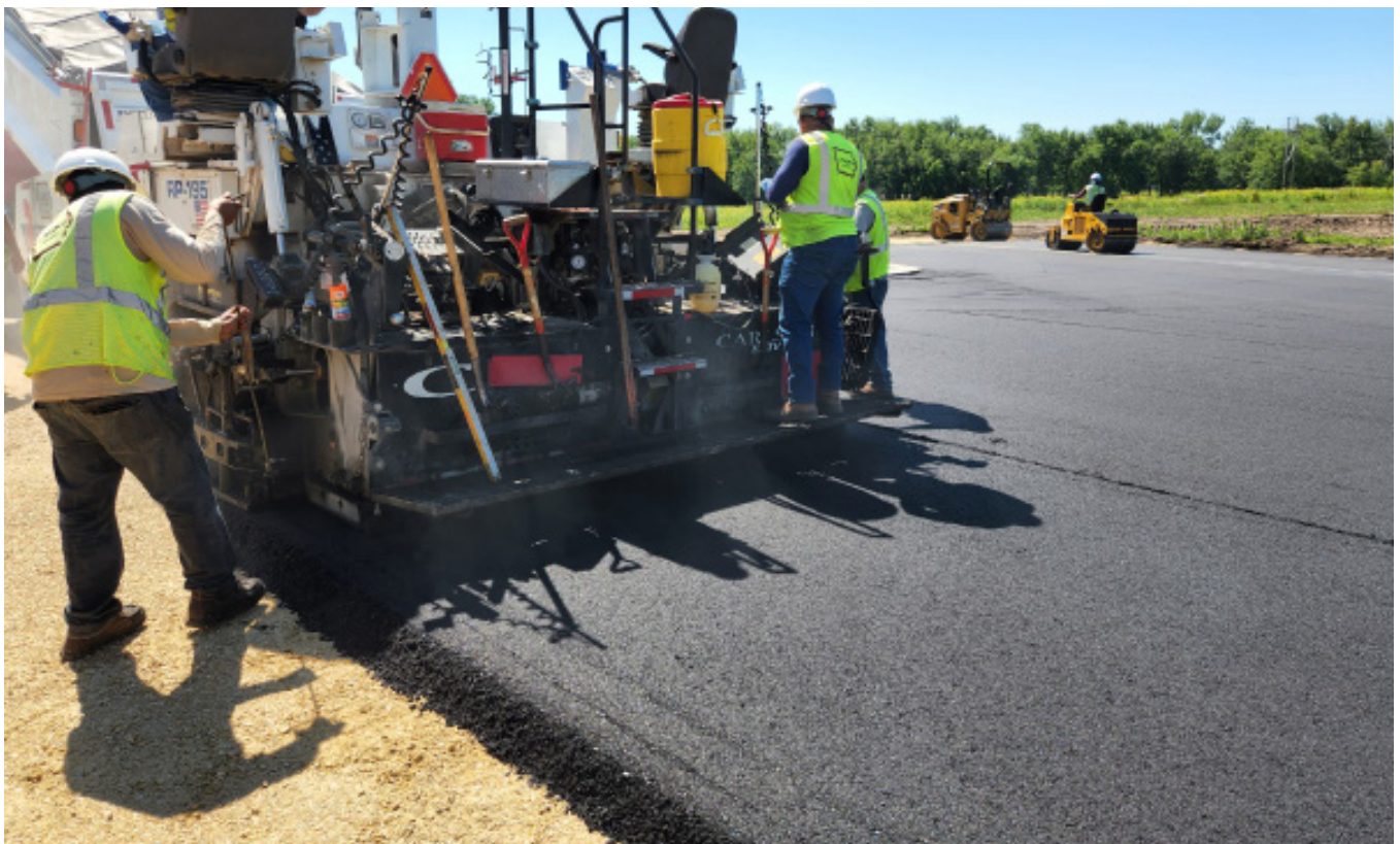
Photo: Paving at the Cedar River Crossing & Sutliff Bridge West Side Improvement Project
