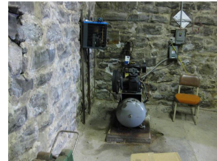
Basement boiler room.
