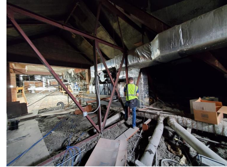
Ductwork in attic.
