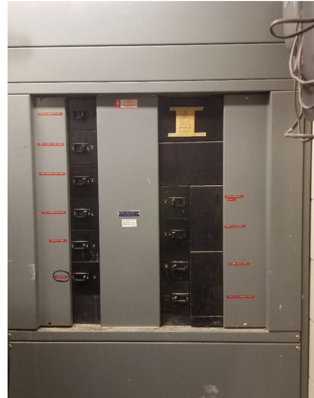
Main distribution panel.
