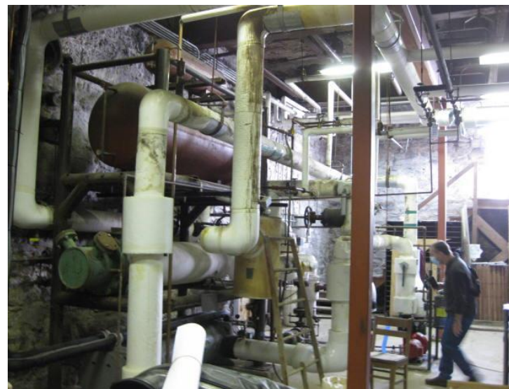
Basement boiler room.
