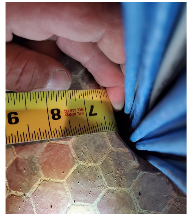
Telecom cables through floor.
