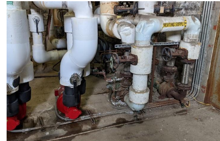
Chilled and heating water pumps.
