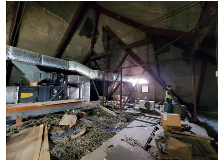
Ductwork in attic.
