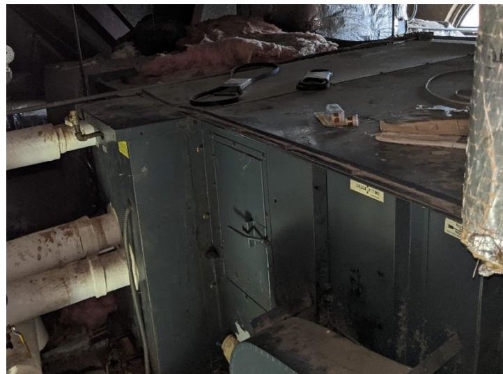
South air handler in attic.
