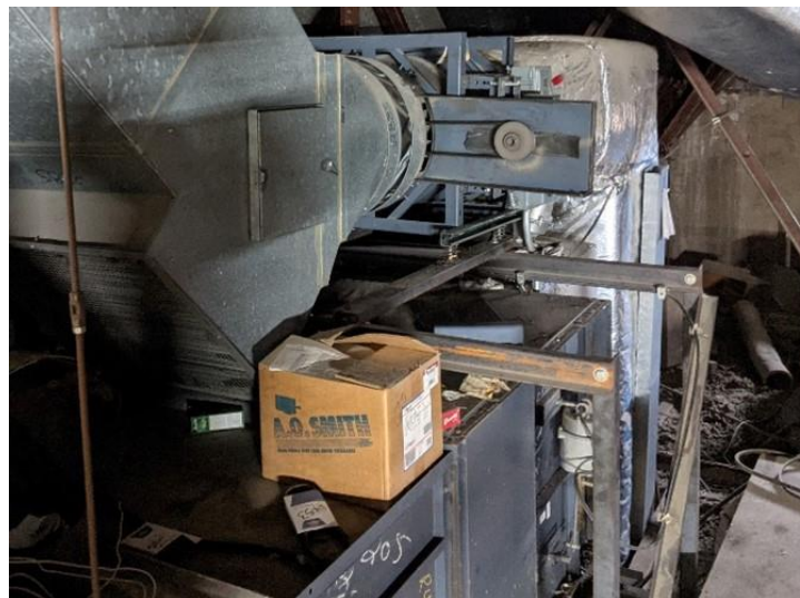
North air handler in attic.
