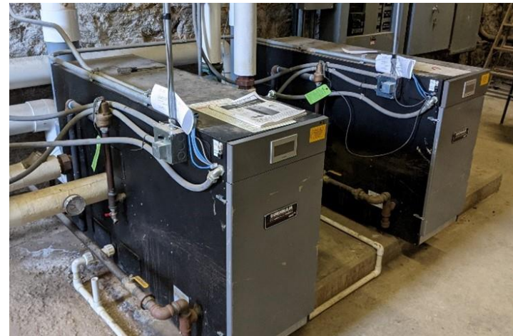
Boilers in annex.
