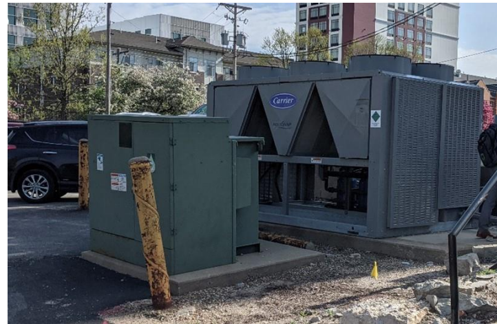
Existing chiller and annex transformer.
