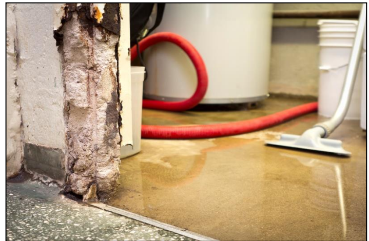
Flood or sewer backup
